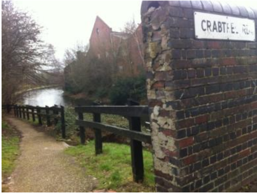
Re-graded ramped access to Birmingham Canal Old Line towpath, sealed aggregate surface (but requires widening and removal of overhanging branches to bring up to cycle route standard)
