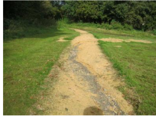
Eroded gravel path on slope in Selly Oak Park. Sealed surface is more expensive but may have reduced overall costs when maintenance is considered
