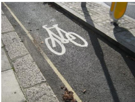
Kerb separated cycle track width should be 2.0m to allow for sweeping and overtaking, chamfered kerbs would be more forgiving than right angled kerbs.
