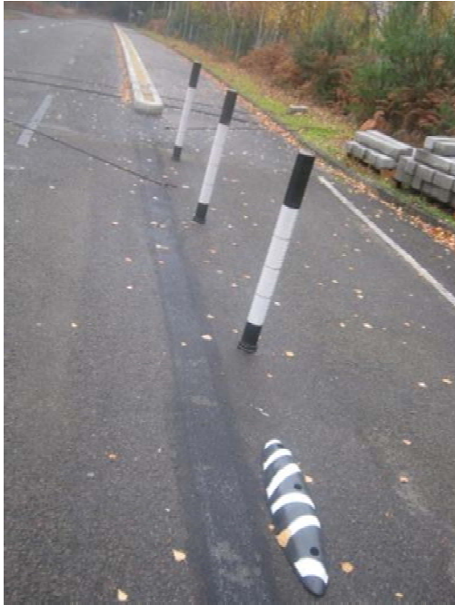
TRL test site for separation using Zicla Zebra, Wand bollards, and kerb separation for a cycle track.
