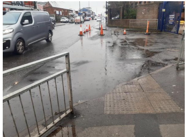
7.1 Puddling and damaged surface across wide entrance
