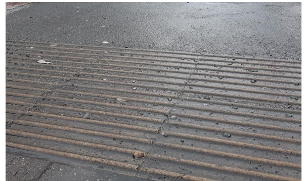
4.3 Broken glass on footway of the alternative route to the main entrance (at bus stop)
