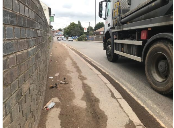
2.2 Build up of debris on pavement opposite station
