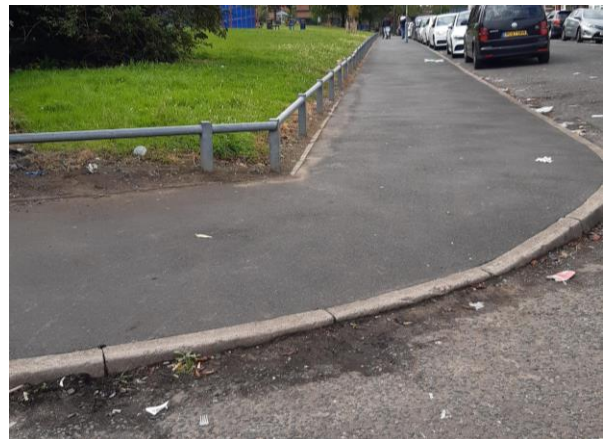
6.2 Dropped kerb not flush at end of Denbeigh St. People with wheelchair seen finding this difficult, having to go up it backwards.
